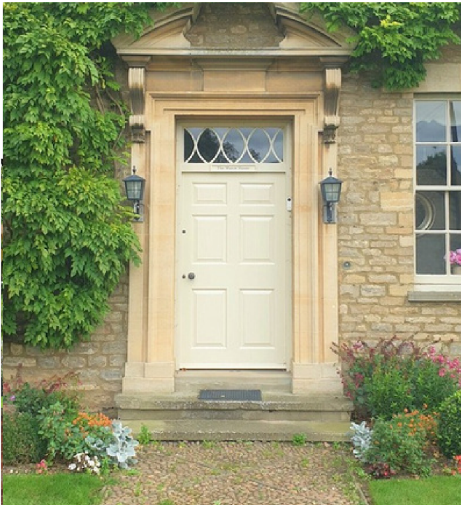
Door at The Manor House, High Street. The house has origins in the C17th; this is a 6-panel door divided by a horizontal frieze rail and a locking rail and then divided vertically by central 'muntin' boards. There is a shouldered stone door surround, itself contained within shallow pilasters, topped by fluted, consoled brackets, supporting a broken segmental pediment above. The ornate glazed fan, or transom light, is above the door. The door itself is only occupies a relatively modest proportion of this grand composition.
